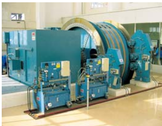
▼ Mine hoist motors
